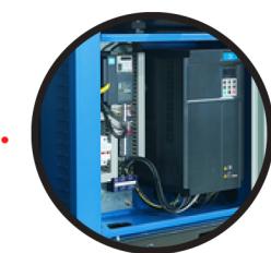
VSD Controller for Main & Fan Motor
